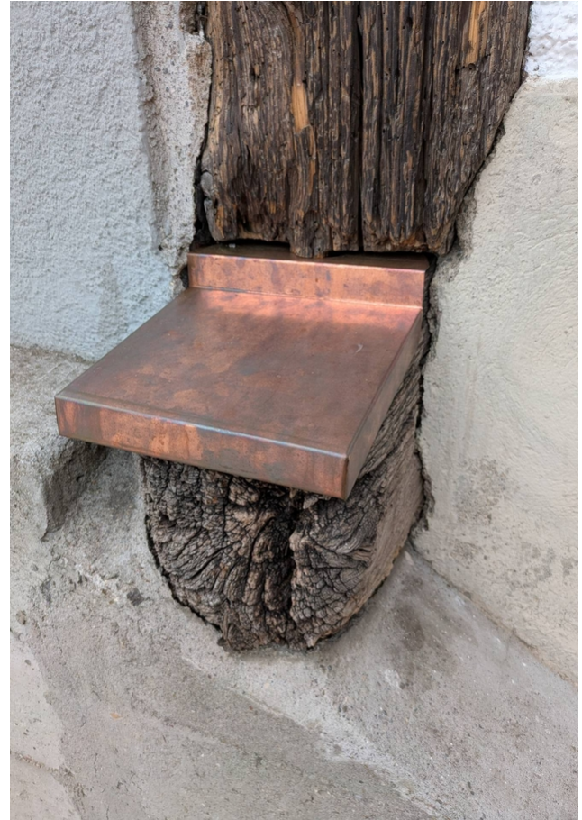
Constructive wood protection helps to protect the half-timbered structure from moisture penetration.
